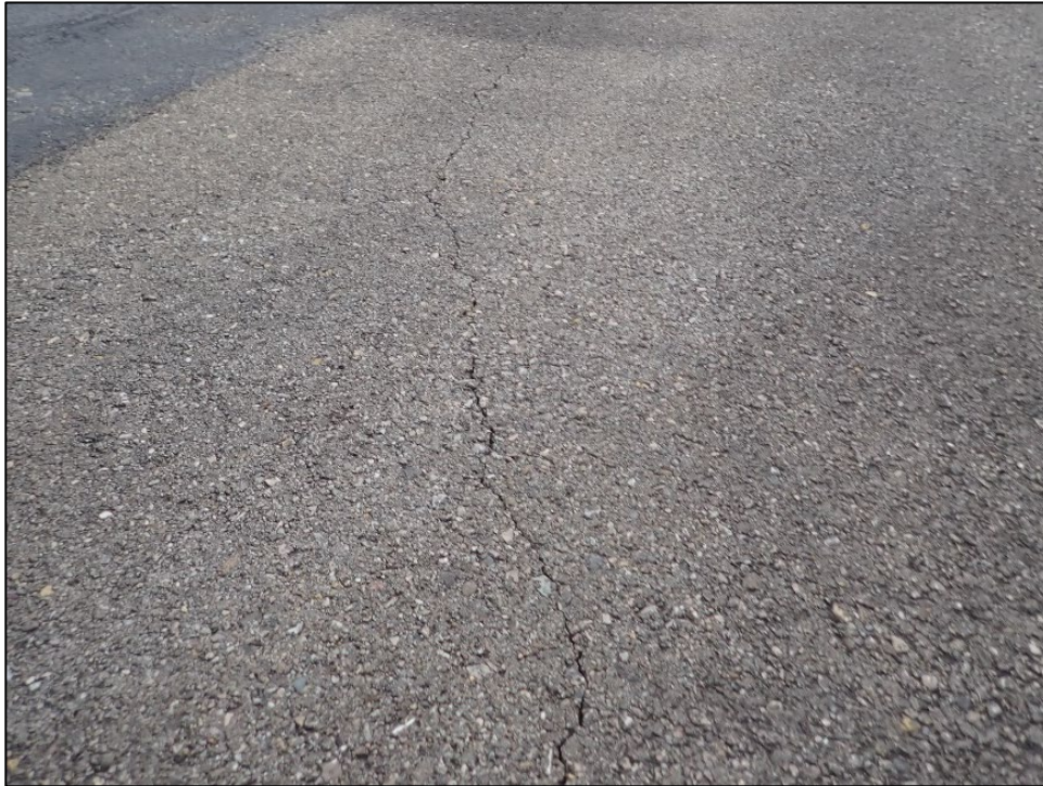
AP-21-05: L&T Cracking
