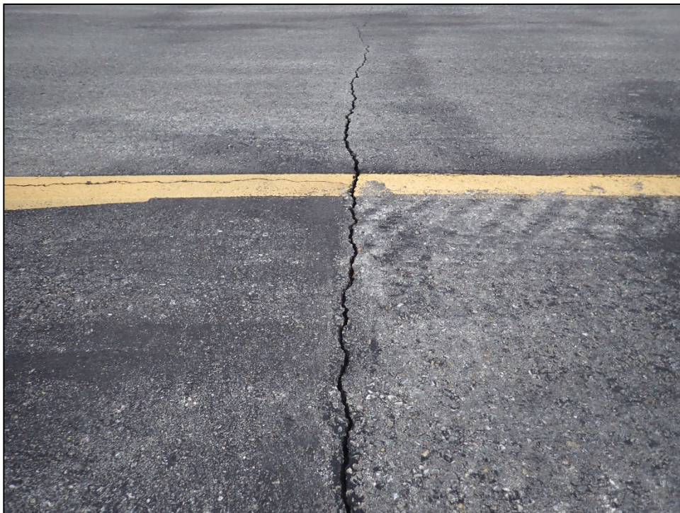
TW-21-10: L&T Cracking
