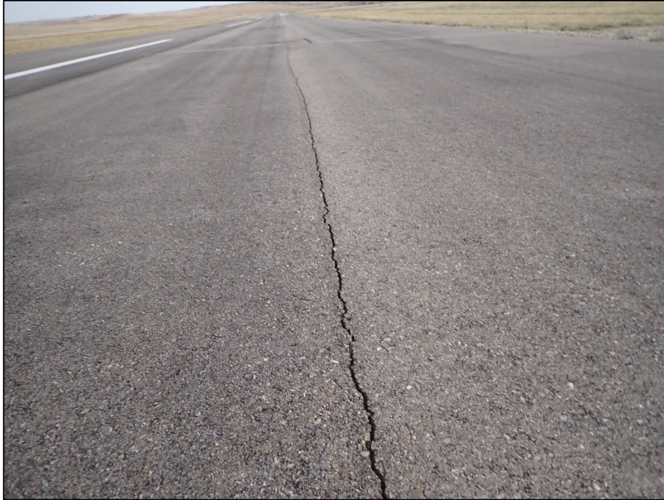
RW09-21-05: L&T Cracking
